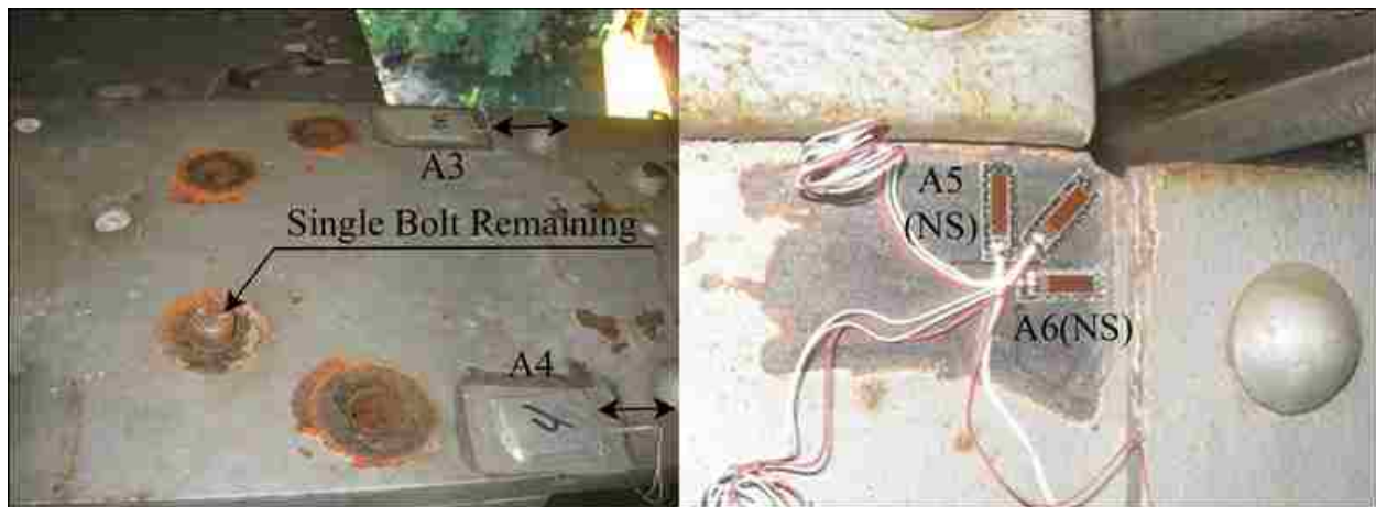
Figure 2-8: Strain gages installed on the tie plate (A3, A4) after 7 of the 8 bolts removed and on the cantilever bracket web (A5, A6)
